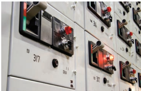
Power generation and distribution.
