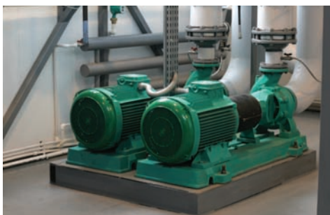
HVAC, pumps and valves.
